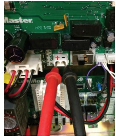
Figure A Testing motor connection on the Logic Board
